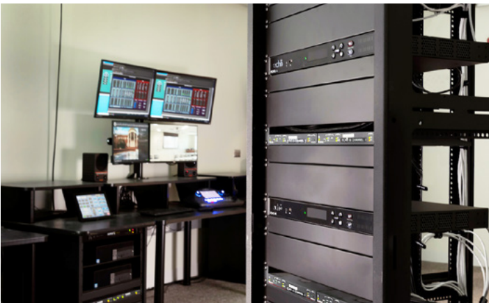
The use of the NAV Pro AVoIP system cut the rack load from three full racks to half of a single rack. In addition to space savings, this greatly reduced the heat load within the DE control room.
