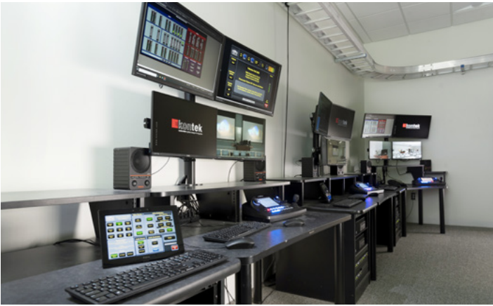
Each camera and microphone throughout the building ties back via NAV to the operator stations within the DE control room. This enables remote monitoring, audio mixing, and control.
