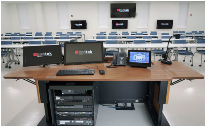
Rack-mounted within the instructor lectern located in each active learning and traditional classroom is the AV system. It includes NAV E 101 encoders and NAV SD 101 scaling decoders. Additional scaling decoders are mounted to the two projector lifts.
